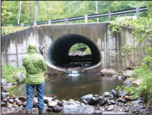
The Beartown Road culvert in Underhill is one of the culverts considered for a retrofit.
