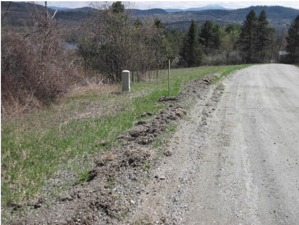
Figure 22: Project 21 – Mount Pritchard Lane improvements
