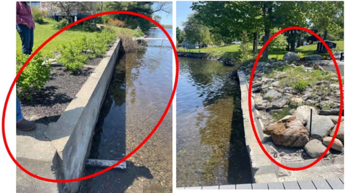
Figure 14: Project 12 – Sea wall removal and bank restoration along Pine Shore Drive (photo from WNRCD)
